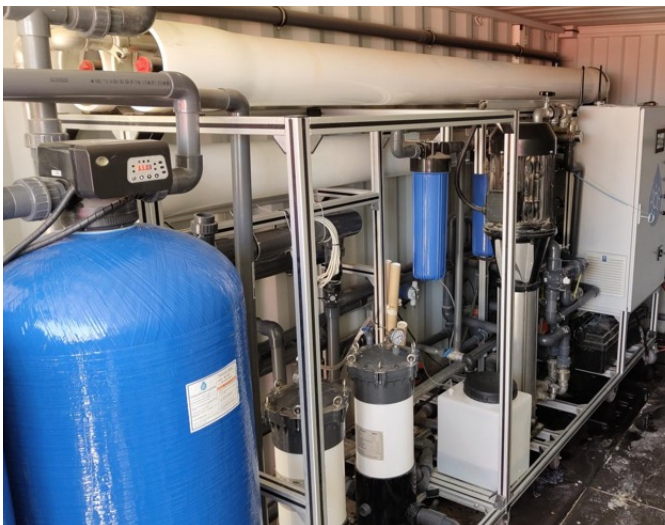
Reverse-osmosis desalination skid inside a containerized unit, with pre-filtration, RO membranes, pumps and dosing equipment. Credit: Oxfam.
