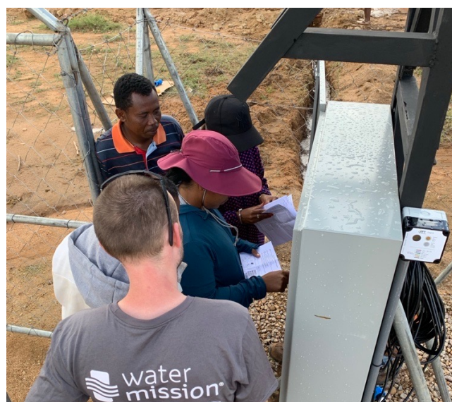
After the first installation, training the local UNICEF staff about its operations and maintenance. Credit: Derek Chitwood.
